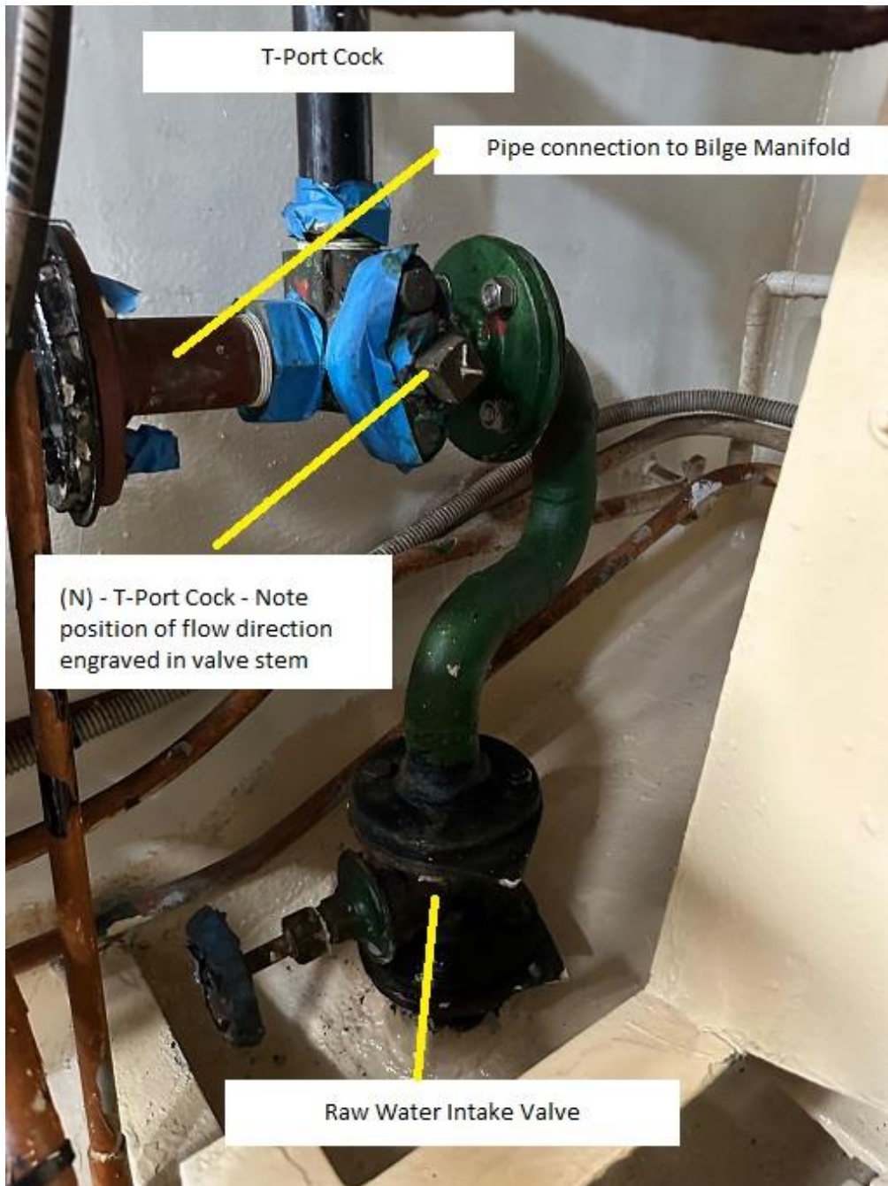
IMAGE 7 -T-PORT COCK CONNECTION TO BILGE MANIFOLD
